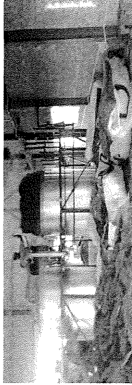
Picture below shows Ezingoleni Tee Tree Distillery Plant.
